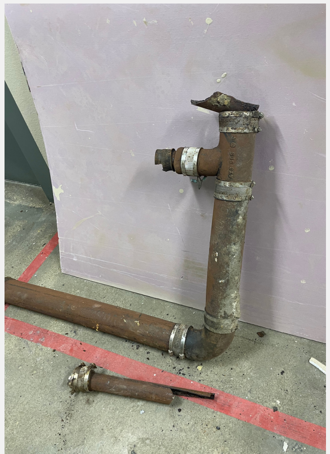
Corroded pipe being replaced
